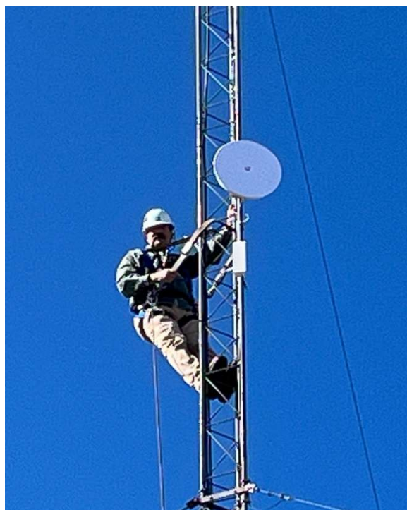
N7MSI on the tower with the Internet link antenna (top) and AREDN antenna (lower).
